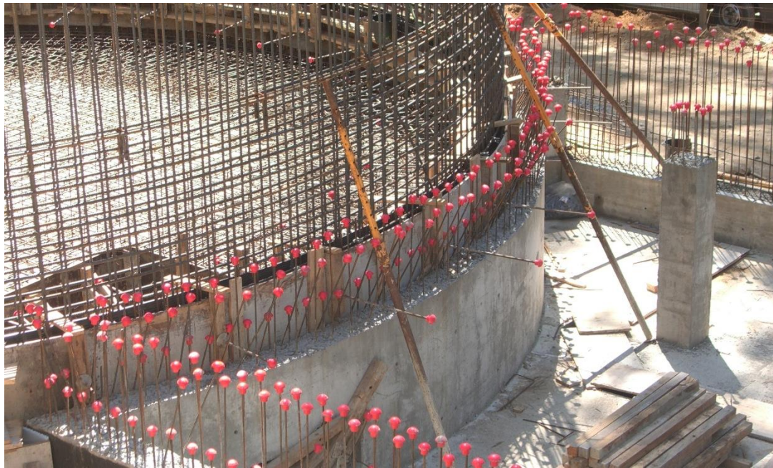
FIGURE 3: PROTRUDING REINFORCEMENT STEEL WITH PROTECTIVE ENDCAPS.
