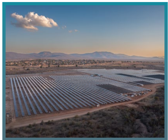
The Bolobedu power plant in South Africa, whose annual output is expected to prevent the emission of more than 237,000 tons of CO 2 .
